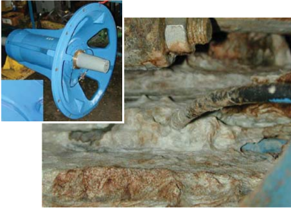
LabTecta-TE-OAP™ installed on a hydropulper gearbox in 2006 (Case Ref: 3327).
