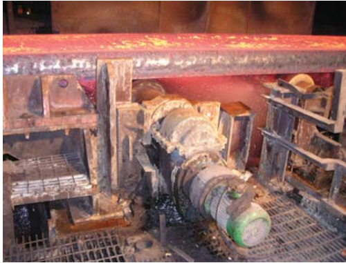
Leaking gearbox creating a fire hazard in a steel processing plant.
