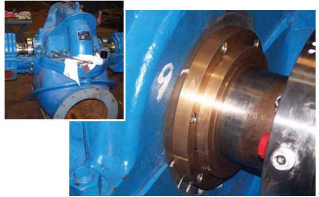
Flange mounted LabTecta-RDS™ installed on a double-ended pump in 2007 (Case Ref: 3304).
