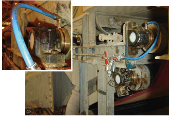
Multiple LabTecta-PB-OAP™ installed on a conveyor belt in the mining industry in 2006 (Case Ref: 3317).
