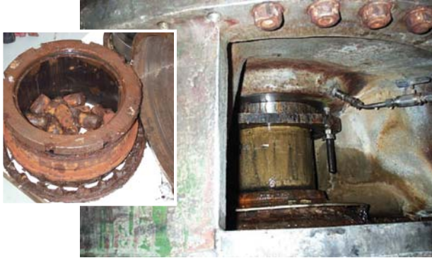
Water contamination on a continuous digester prior to a LabTecta™ being installed (Case Ref: 3232).
