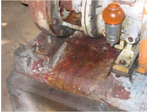
Over-filled unbalanced lubricator presenting undue failure risk.
