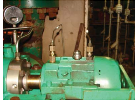
Sulzer MSD BB3 pump with MagTecta-OM-AX™ installed in 2006 (Case Ref: 3453).
